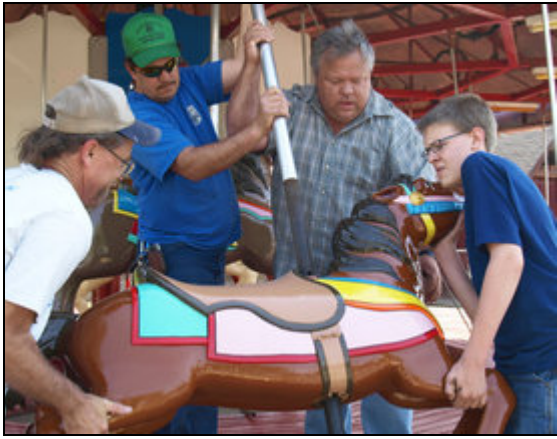
Tim Branch, Jerry Sanders, David Lea and David Turinetti install a newly painted horse on the carousel at Kiddie Park in Bartlesville.
